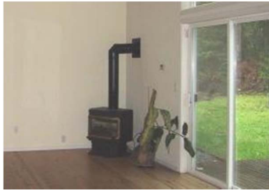
Original Propane stove
